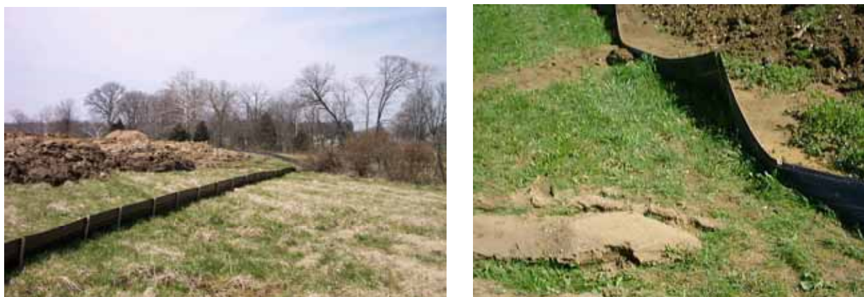
FIGURE 5-7 A functioning silt fence (left) and an improperly maintained silt fence (right). SOURCES: EPA NPDES Menu of BMPs and Robert Traver.
