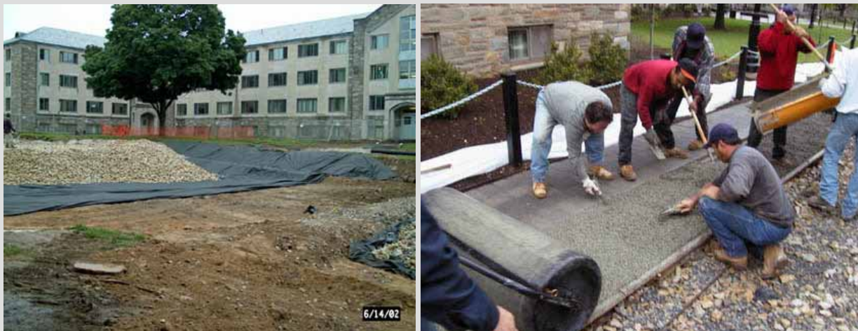
FIGURE 5-34 Infiltration bed under construction. Pervious concrete has functionality and workability similar to that of regular concrete. However, the pervious concrete mix lacks the sand and other fine particles found in regular concrete. This creates a significant amount of void space which allows water to flow relatively unobstructed through the concrete. This site was the first attempt at creating a pervious concrete SCM in the area, and there were construction and material problems. Since that time the industry has matured, and a second site on campus constructed in 2007 has not had any significant difficulties. SOURCE: Reprinted, with permission, from VUSP. Copyright by VUSP.
